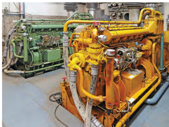
Standby generators . Photo Clive Penfold
